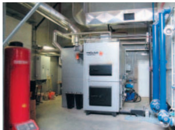
Figure 32: Biomass boiler with 200 kW. Source: BE 2020+, 2010.
